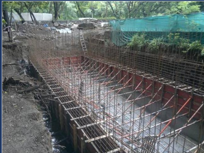
Fire hydrant tank of 5 Lakh Litre for Cummins India Ltd.
